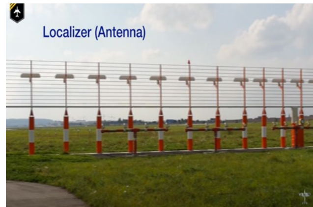
Fig.1. The Localiser Antenna Subsection
