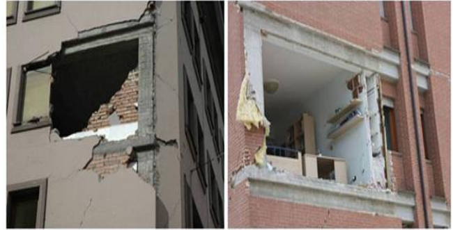
Fig.5. Examples of out-of-plane collapse of infills poorly connected to the RC frame
