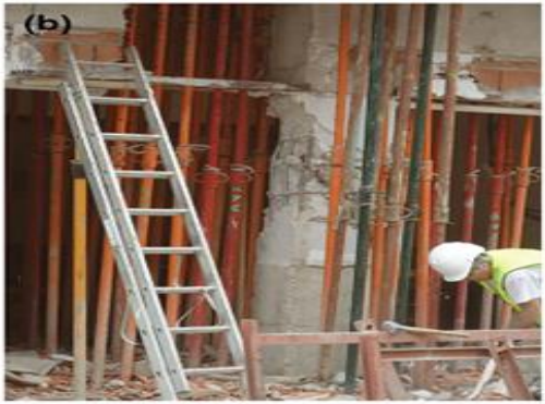
Fig.7(b). Severely damaged column
