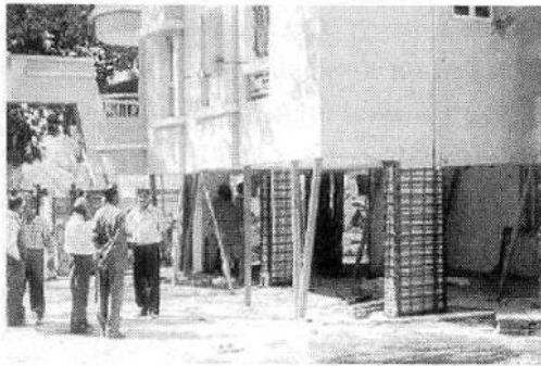
Fig.1(a). Precariously balance severely damaged RC frame buildings with open ground storey in Ahmadabad
