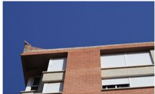
Figure.6. Building with a partially collapsed parapet wall
