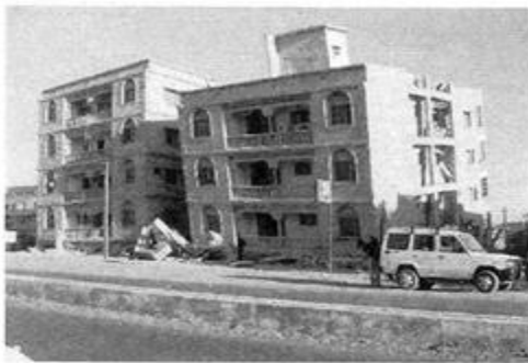
Fig.1(b). Ground storey collapse of a four storey building with open ground storey at Bhuj
