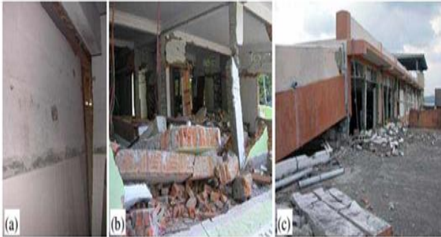
Fig.3. shows OOP failure of masonry infills in buildings at (a) Mohanpura (school building), (b) Bamboo flat, and (c) Passenger Terminal Building at Haddo wharf.
