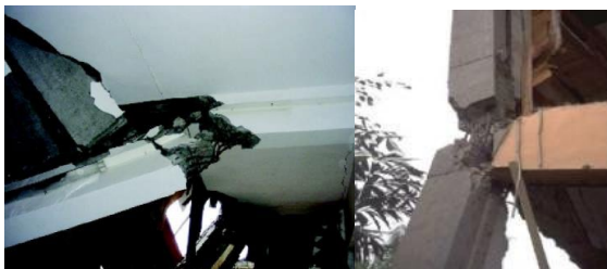
Fig.4. Beam and Joint Failure during Earthquake Source: Research Gate – Patnaik et.al (2012)
