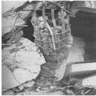
Fig.1. Damage on top of first storey columns after Moro Gulf Earthquake
